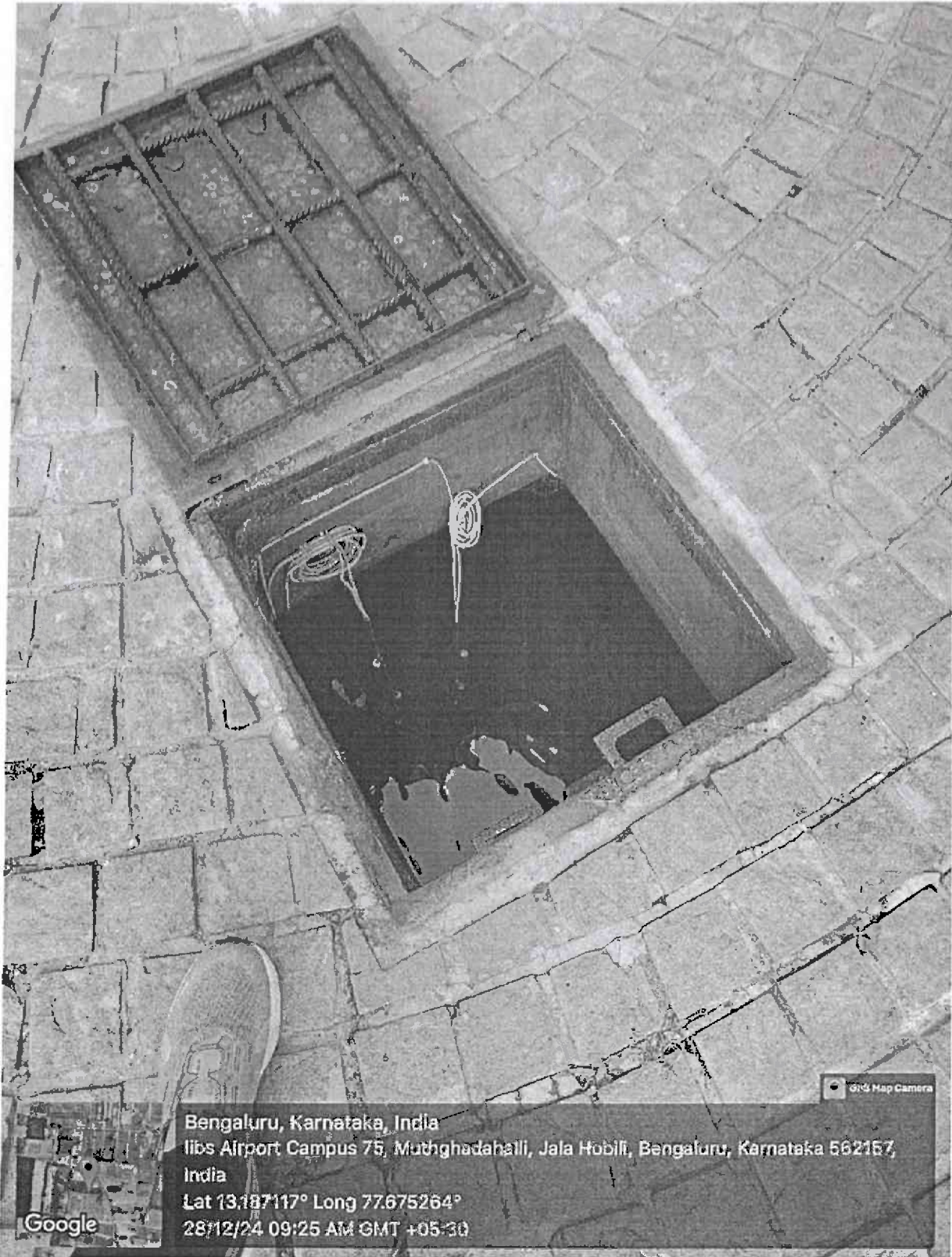
Bore well /Open well recharge
